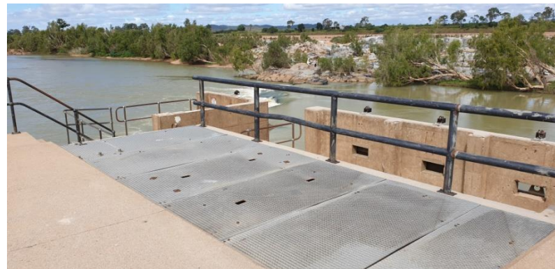
Burdekin River and Rocks Pump Station Pump intakes.
