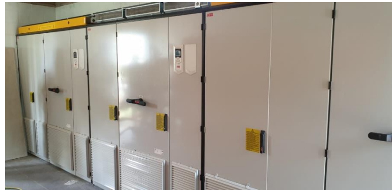
Installed ACS880-37 variable speed drives.
