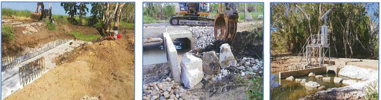
Figure 7: Capital works infrastructure project: Construction of the Saltwater Creek automated water control gates, channel crossing and fish ladder.
