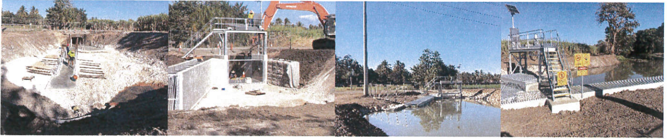
Capital Infrastructure Project: Cislowski Road automated gate and fish ladder during and after construction
