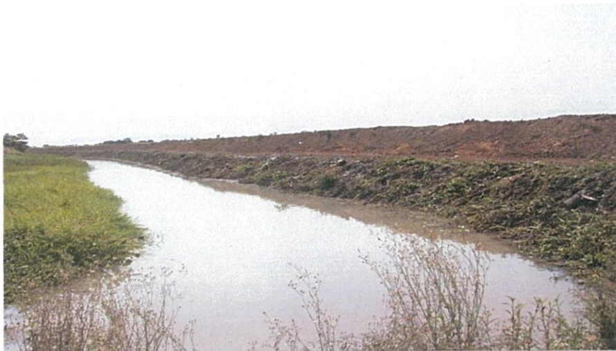
Water Distribution Channel
