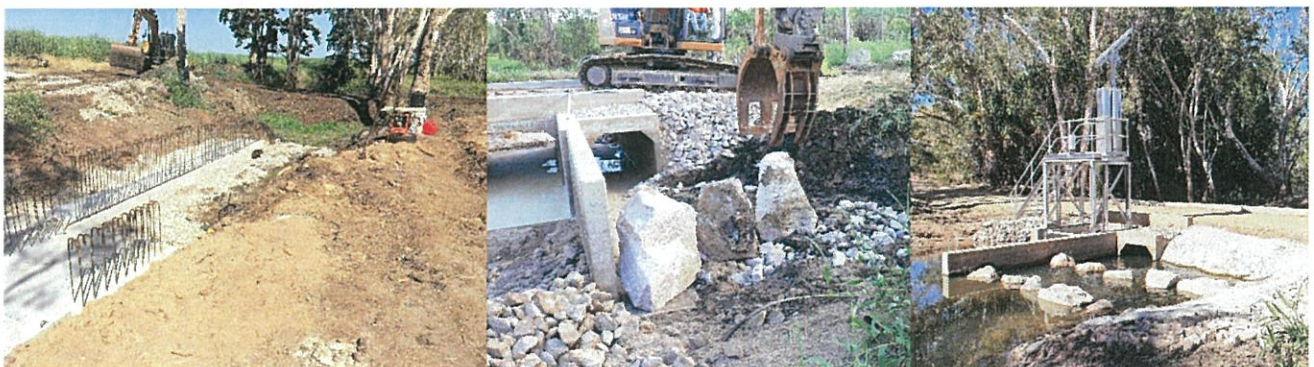
Capital works infrastructure project: Construction of the Saltwater Creek automated water control gates, channel crossing and fish ladder.
