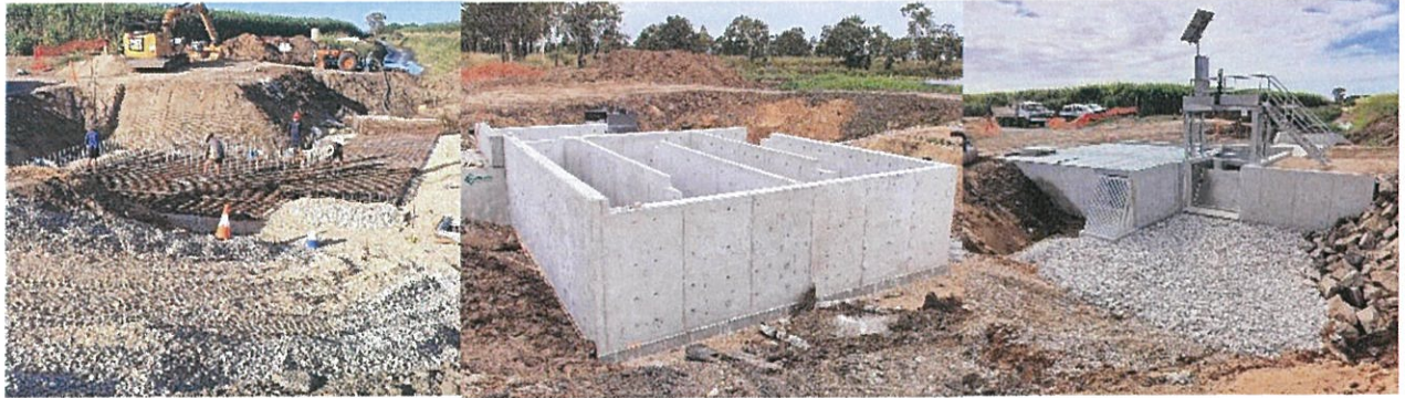
Capital works infrastructure project: Construction of the Rocky Ned Road automated water control gates, channel crossing and fish ladder.
