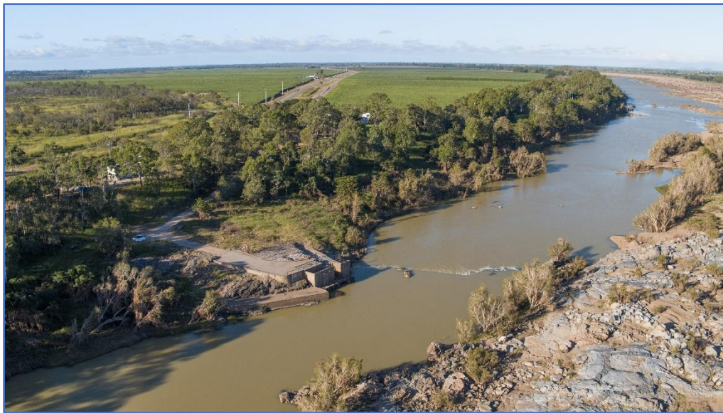
Figure 5: The Rocks Pumpstation on the Burdekin River
